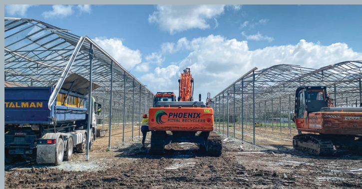
Above: Favona Glasshouses synchronised glass extraction for Goodman Property’s NZGBC Greenstar Mainfreight site. Below: The glass remains from the Favona Glasshouses for recycling into batt insulation and other local glass products.
